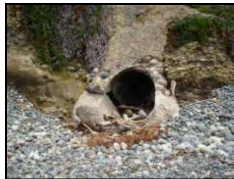
Figure 6. CSD037 (downstream, outlet at Rock Pile Beach, La Jolla)
